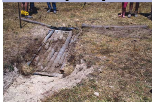
Wiring in the logs
