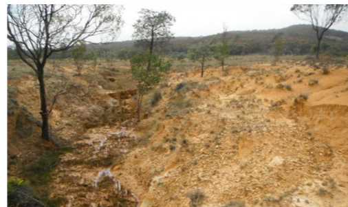
Actively eroding outer bed. Works can help vegetation establishment and halt the lateral migration of the channel.
