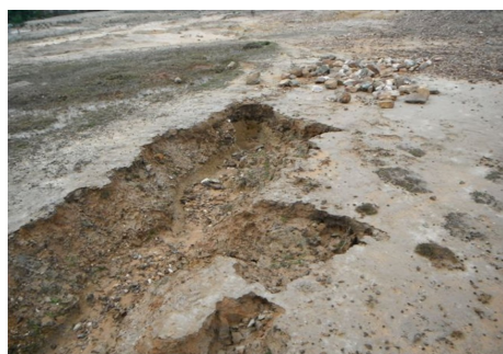
Small gullies like this which threaten access can easily be halted with simple works.
