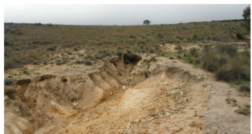
Headcut moving up a 1 st order valley. Not a particularly high priority unless infrastructure is threatened, but sediment delivery can be reduced.
