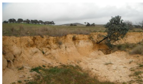
Actively eroding outer bed. Works can help vegetation establishment and halt the lateral migration of the channel.
